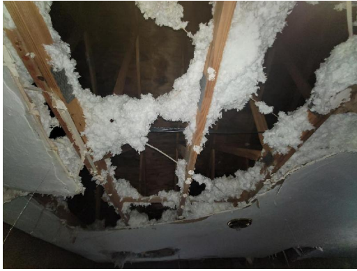
Interior Living Room Southwest drywall ceiling, insulation Visible water damage Visible microbial growth
