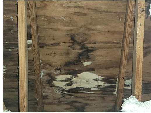
Interior Living Room Wood framing, wood roof decking Visible water damage Visible microbial growth
