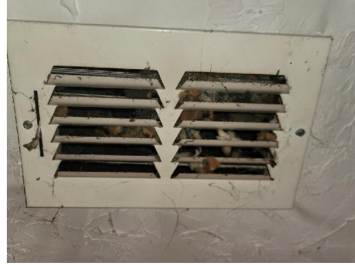
Interior Northeast Bedroom Metal HVAC ceiling vent Visible debris Visible microbial growth (Observed at multiple Interior locations)
