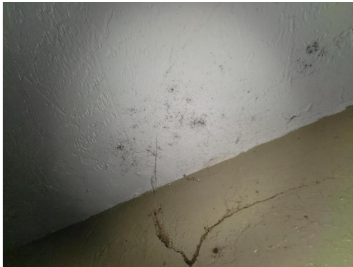
Interior Southeast Bedroom Drywall ceiling, drywall upper wall Visible water damage Visible microbial growth
