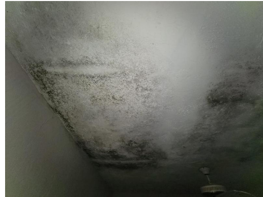
Interior Northwest Bedroom Drywall ceiling, drywall upper wall Visible water damage Visible microbial growth
