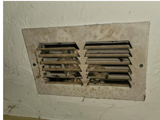
Interior Southeast Bedroom Metal HVAC ceiling vent Visible debris Visible microbial growth (Observed at multiple Interior locations)
