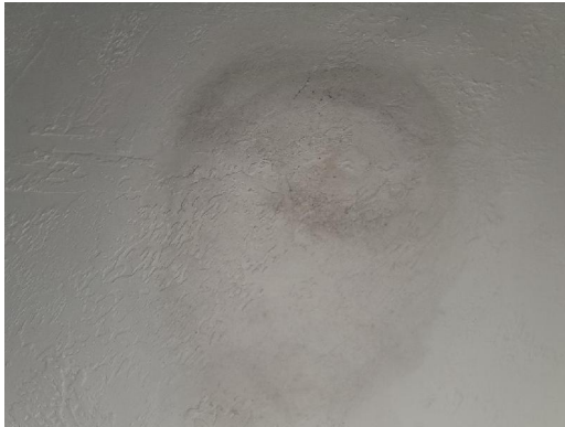
Interior Southwest Bedroom Drywall ceiling Visible water damage Visible microbial growth
