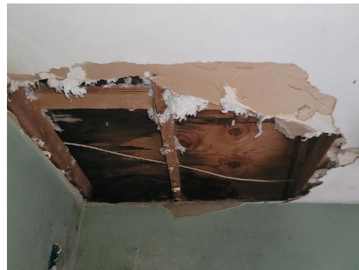
Interior Rear Entry Drywall ceiling, drywall upper wall Visible water damage Visible microbial growth
