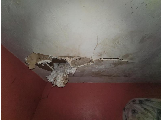
Interior Northeast Bedroom Drywall ceiling, drywall upper wall Visible water damage Visible microbial growth
