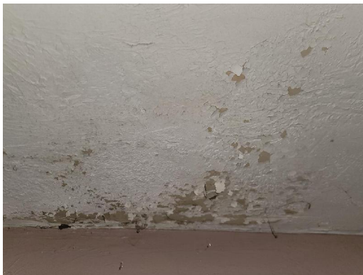
Interior South Bedroom Drywall ceiling Visible water damage Visible microbial growth
